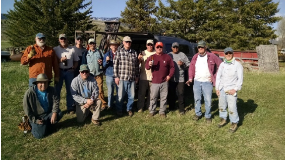
Fence deconstruction crew, celebrating at the end of a long and very productive work day.
